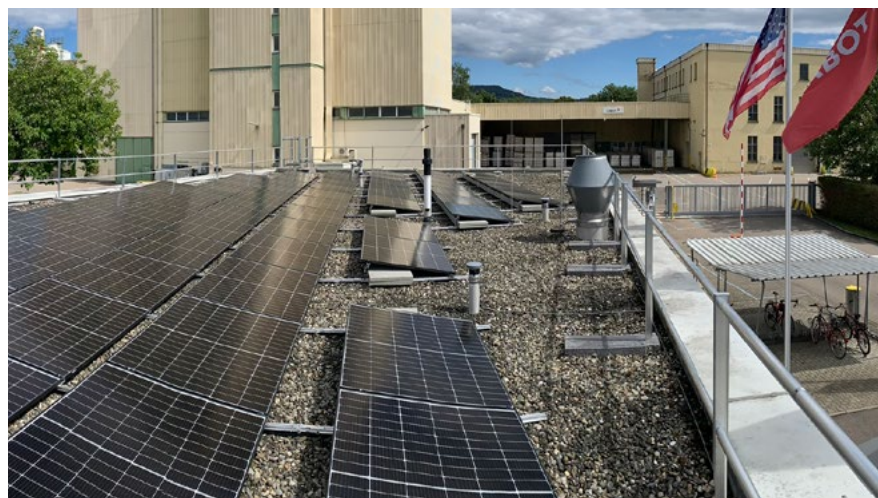
Solar array on roof in Rheinfelden, Germany
